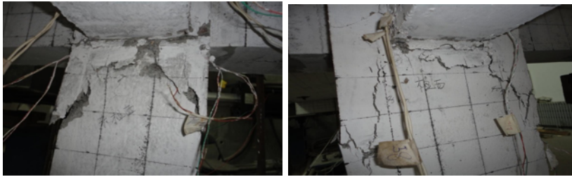
Fig. 8. Failure mode of specimen KJ-1
