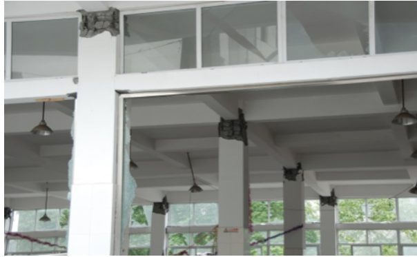
Fig. 1. The column hinge failure of frame structure in Wenchuan earthquake
