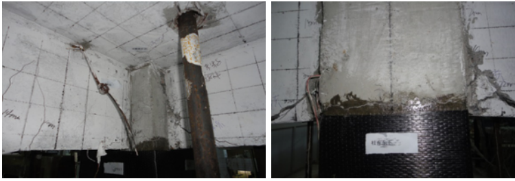
Fig. 9. Failure mode of specimen KJ-1
